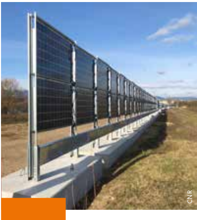
The Compagnie nationale du Rhône (CNR) has commissioned a demonstrator with vertical bifacial modules on the Sablons dyke (Isère). It is deployed over 350 metres with 104 kW of installed capacity. These 3-metre high panels are more resilient and watertight than classic ground-based PV panels.
